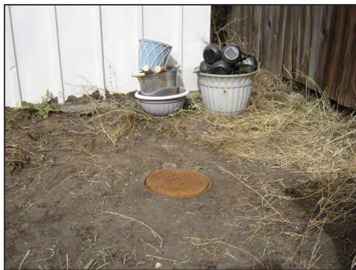
Figure 6 - Cast iron box at ground level.
