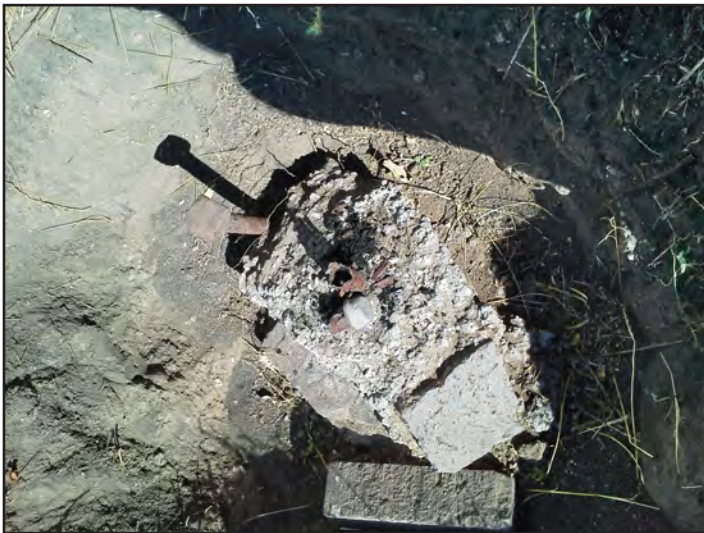
Figure 3 - Concrete cap with pipe and broken off water line brass cap.
