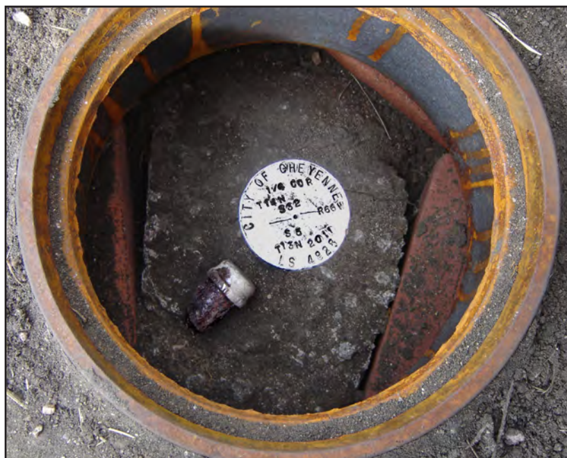
Figure 5 - Reset Aluminum Cap in cast iron box with water line brass cap lying alongside.
